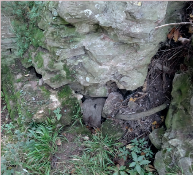
Keep foundations showing the voids
