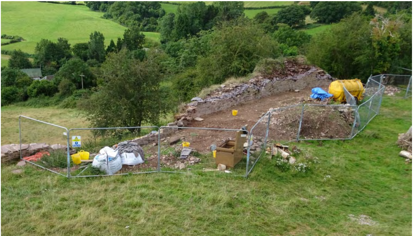
South Curtain wall in July 2019 showing the earth pulled back (and repair work in progress)
