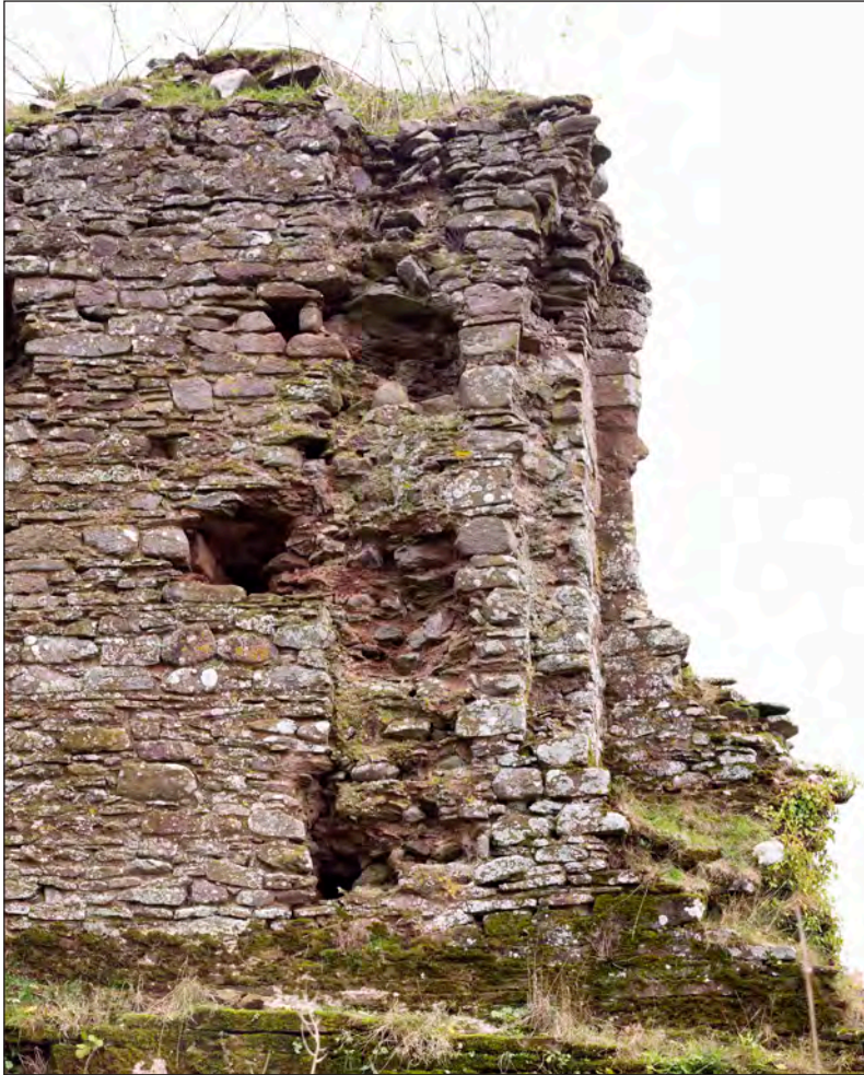
Figure 11 Exposed rubble core, possibly marking the position of a further subdivision in the building (DP195363 cropped).
