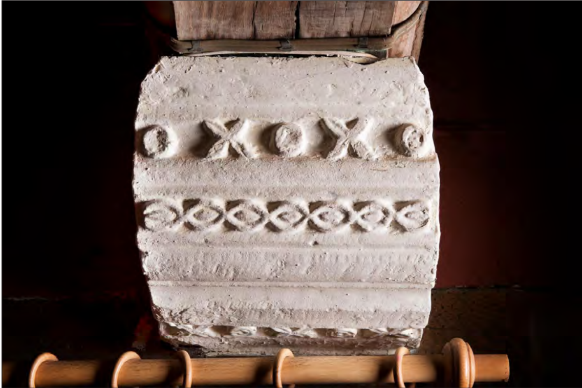
Figure 27 Snodhill Court, one of the corbels supporting the eastern end of the cross beams in the hall (DP195435).
