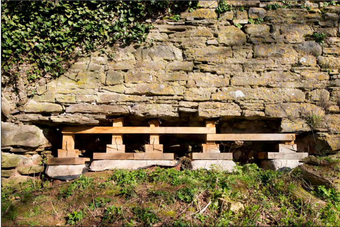
Figure 22 Part of the west section of the south curtain wall, view from south (DP195786).
